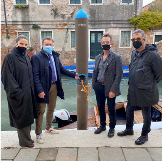
Charging poles have been installed for boats in 'La Serenissima'
