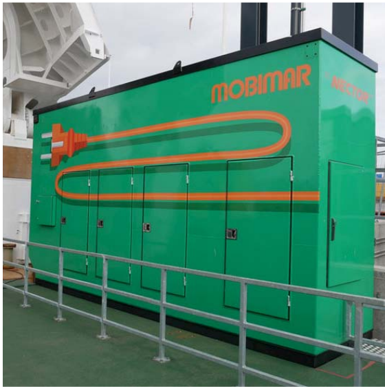
Charging arm of E-Ferry Ellen
